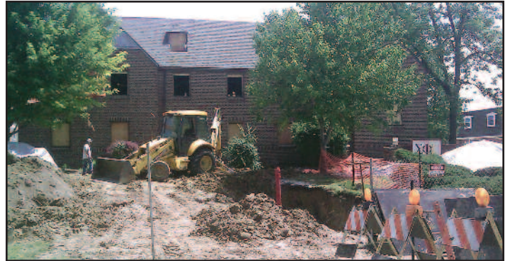
The renovation of 228 Gray is well underway, and construction crews have taken over the property.
