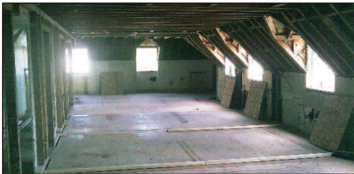
In June, renovations began to make way for the new study suites on the third floor.
